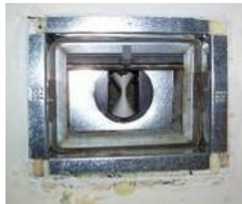
Figure 13. CAR-I damper installed at Echo Apartments(exhaust grille removed)
