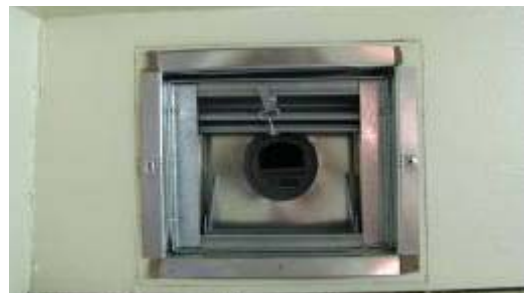
Figure 10– Kitchen Exhaust with CAR-II (grille removed)
