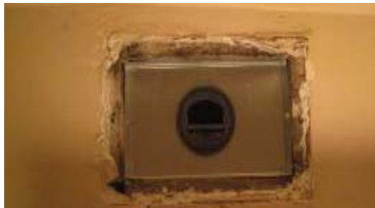
Figure 9– Bath Exhaust w/ CAR-II (grille removed)
