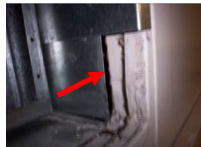
Figure 6. Leakage Area at Connection Between Take-off Duct and Gypsum Board
