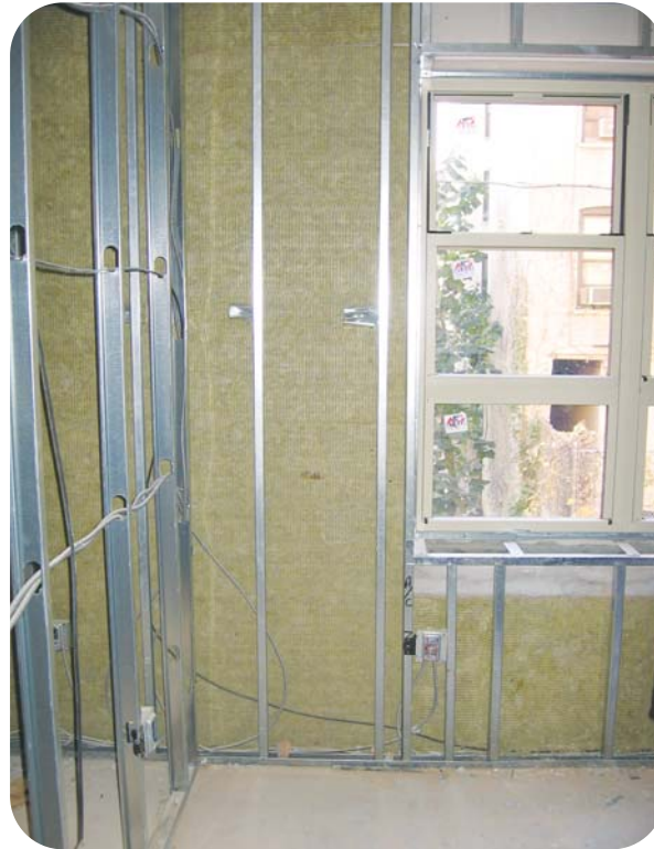
The building walls are insulated with R-4.3 Roxul 1-inch rigid (mineral wool) insulation and R-13 fiberglass batts within 3 1/2-inch interior steel framing. The rigid insulation, placed between the steel studs and the CMU block wall, minimizes thermal bridging through the steel.
